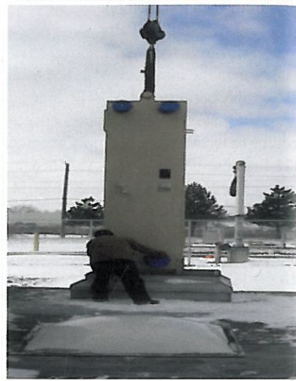
DDI heat exchanger installed in a narrow hatch in Niagara.
