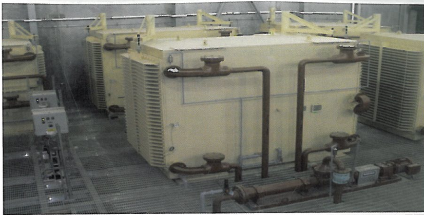
Six heat exchangers in the City of Tulsa, Oklahoma. Two are used as direct-sludge-to-sludge heat recovery; two used as hot water to preheated sludge; two used as cold water cooling the processed hot sludge.
